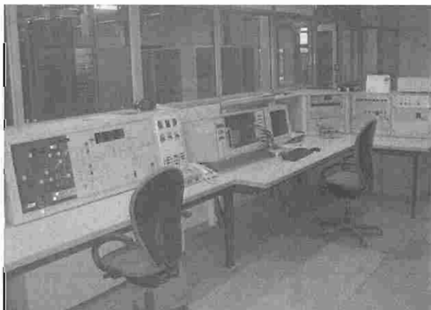
Control station for tests up to 15kA
