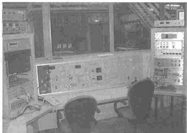
Control station for tests above 15kA
