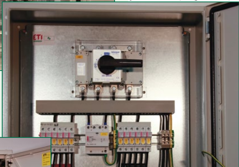
DC junction box (CH gPV fuses)
